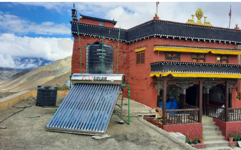
The new thermic solar plant on the mud roof of our living quarters
